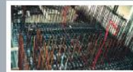
Installation of armoring elements and static armoring elements is performed at the same time
