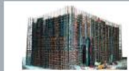
Armoring elements and static armoring elements of a vault room, prepared for panelling and filling with concrete mixture
